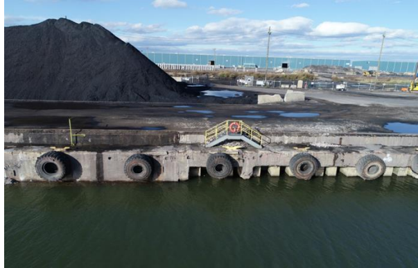
Monitoring system at a crane beam
