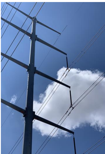
Monitoring system at utility tower
