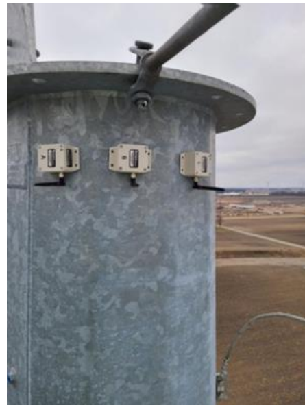
Wireless Accelerometer SenSpot™s on utility tower limbs for vibration monitoring
