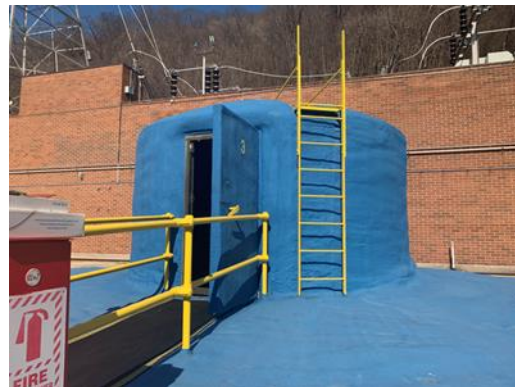
Monitoring system at Hydroelectric Plant (Power Plant Generator)
