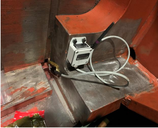
Installed Wireless Strain Gauge SenSpot™ sensors to detect cracks at a structure of a Hydroelectric Plant
