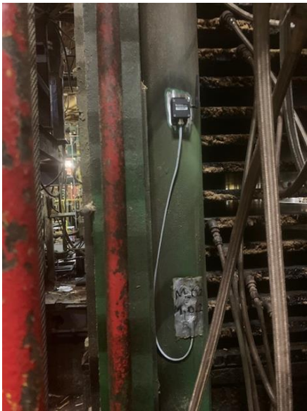
Installed Wireless Strain Gauge SenSpot™ sensors inside a Plywood Factory
